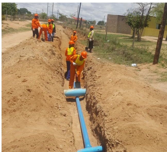
Ceko Water Reticulation Project in Acornhoek, one of the water projects under implementation
