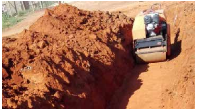
Water Reticulation at Maviljan A, B and C blanket compaction after pipe laying
